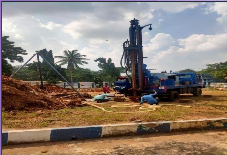
Boring & Casting of Piles work for the construction of Technology Centre, Chennai centre
