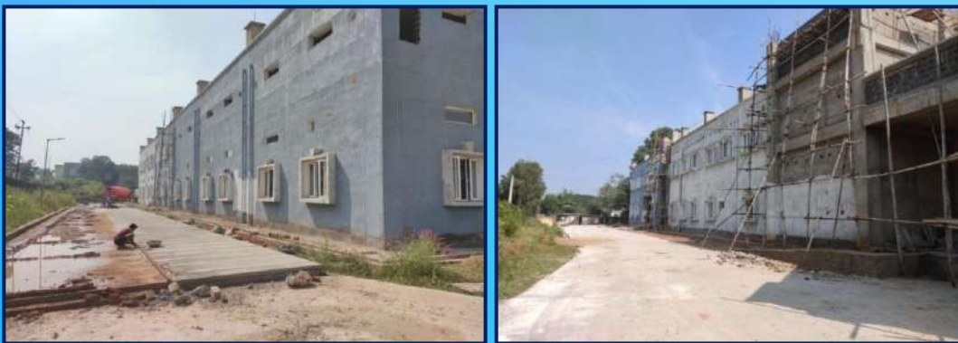
Construction of Academic Cum Workshop Building and Processing Shop Floor at Ranchi centre.
